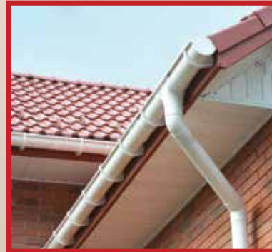
RAIN WATER GUTTERS
